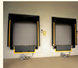
Rolling Service Doors
