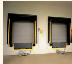
Rolling Service Doors
