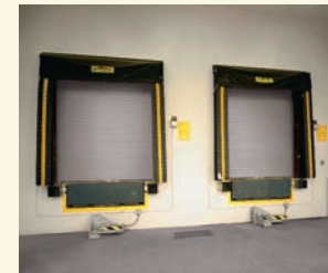
Rolling Service Doors
